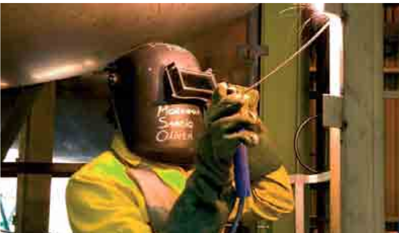
The implementation of a process safety management system was further advanced.
