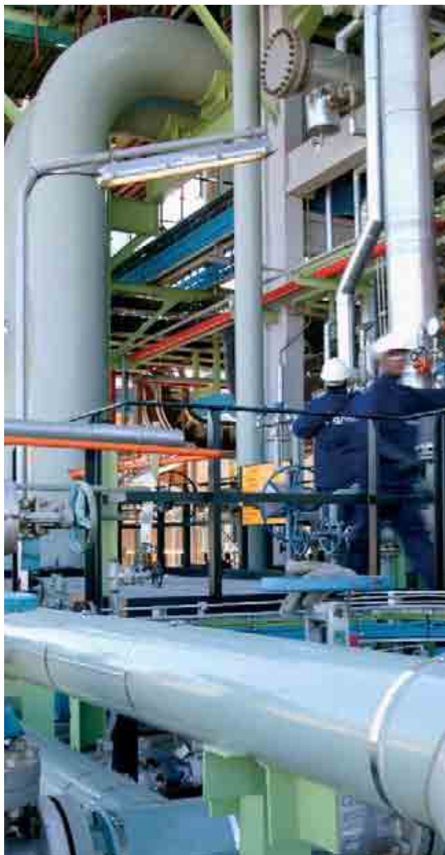
The new Sasol Dia Acrylates plant at Sasolburg in South Africa contributed to Sasol Solvents' record profits.
