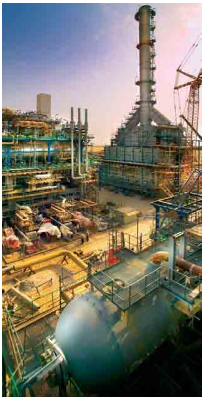
The Oryx GTL plant in Qatar will be brought into production in the year ahead.
