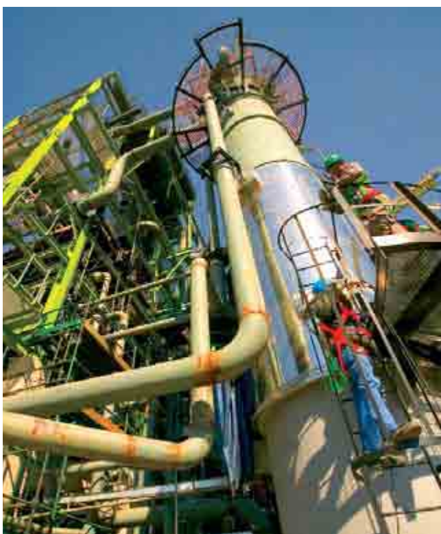
Sasol Synfuels is close to completing Project Turbo at Secunda in South Africa.
